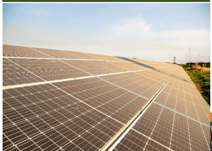
Solar panels generating solar power in the IOM supported Humanitarian Hub in Malakal. Photo Credit: IOM
