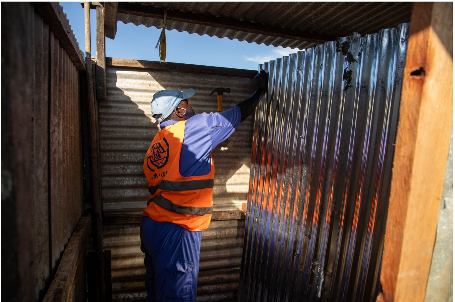
Julia replaces a damaged bathroom door with a new one. Photo: IOM/Nabie Loyce
